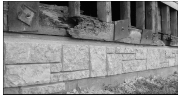
New masonry contrasts with rotten sill that will be replaced in the coming months.
